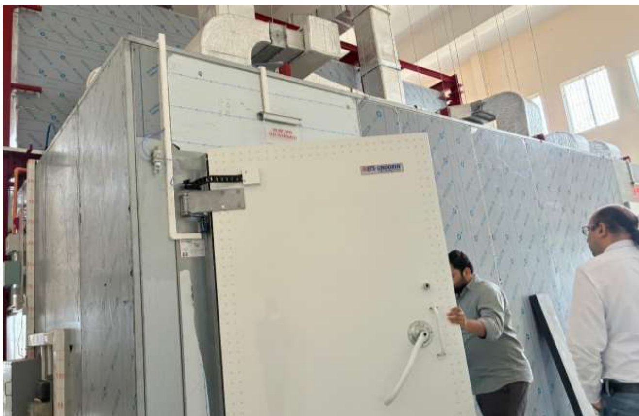
Figure 3.3: EMC Equipment at Medical Device Park CIF Building in Tamil Nadu
