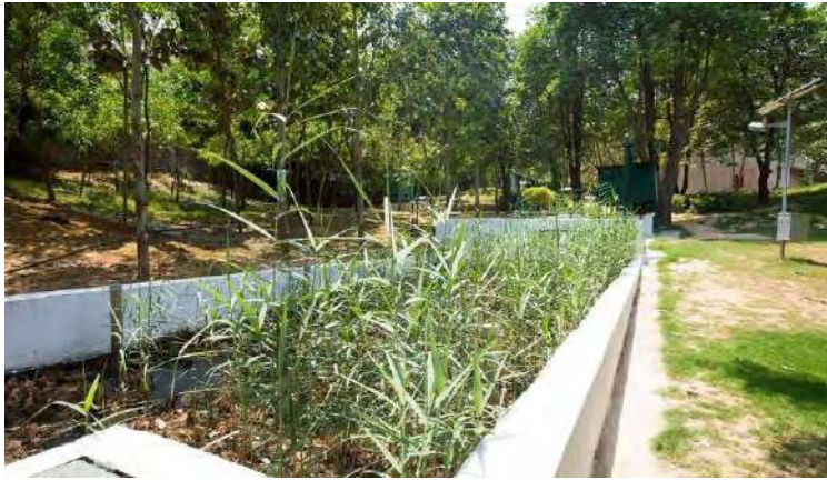
Fig. 2: Phragmites used for treatment of sewage water
